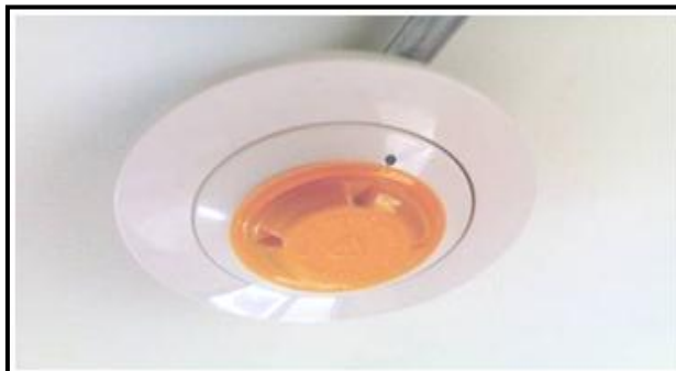
An electric smoke detector
